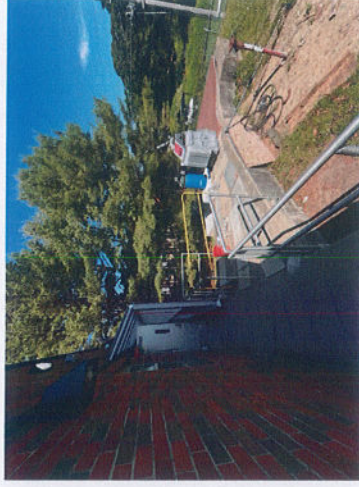
Cover Influent Channels at Headworks
