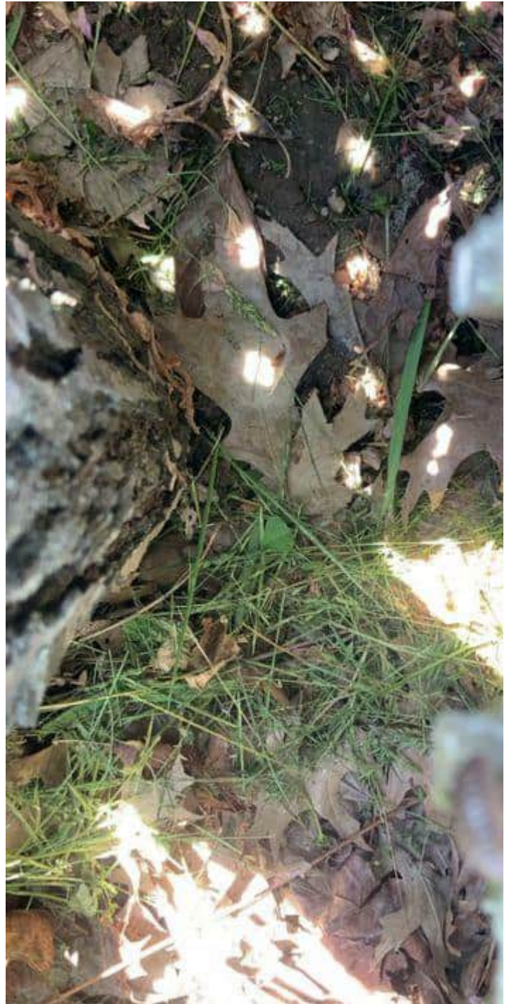
Inside tree box filter
