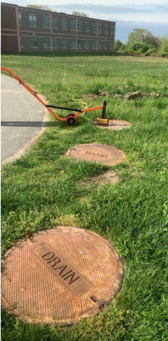
3 manholes of the water quality unit
