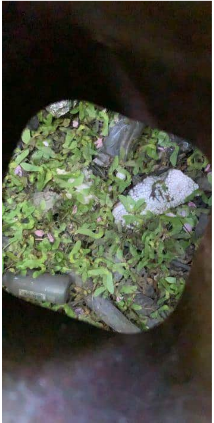
Inside tree box filter
