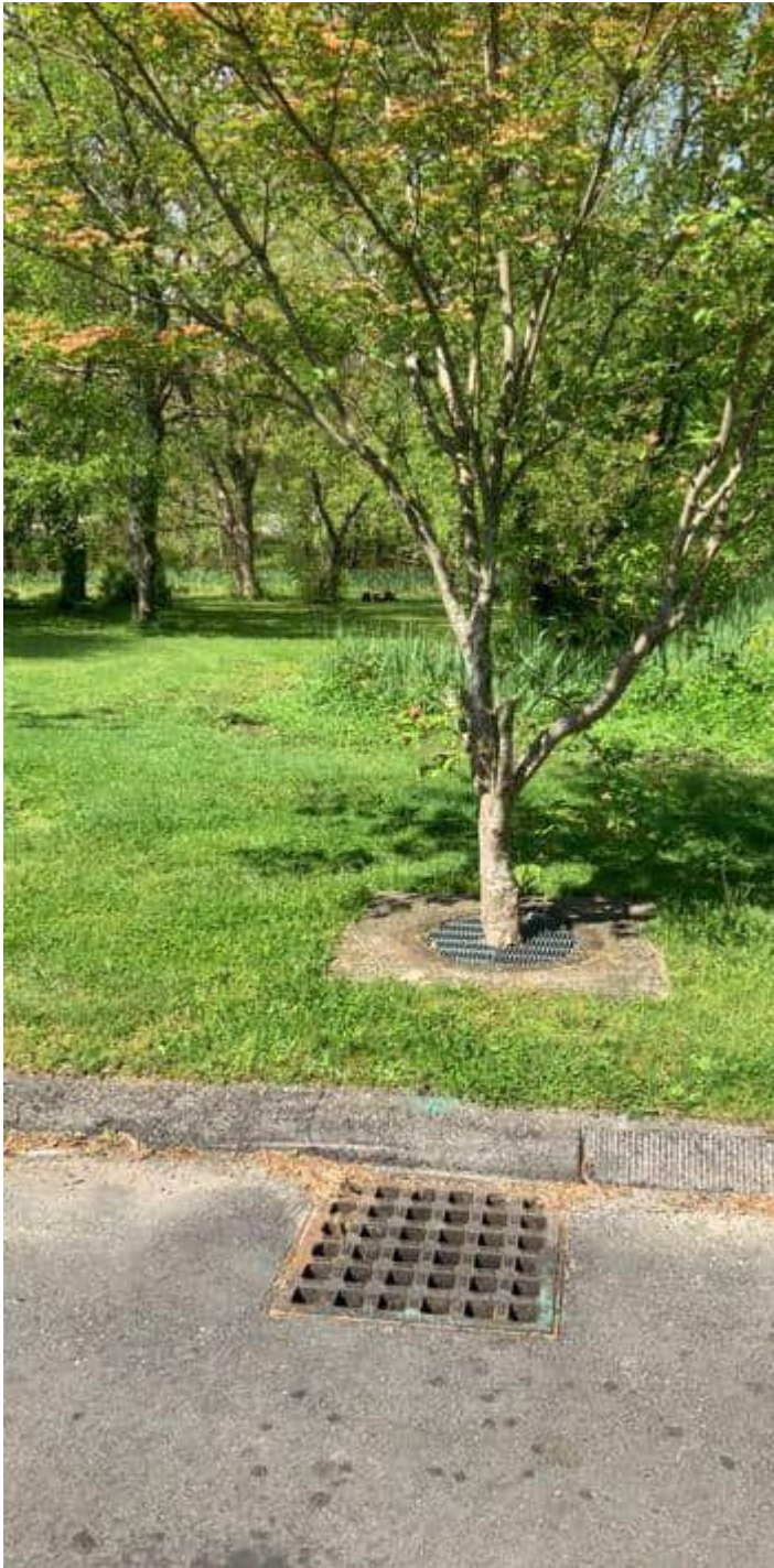
Outside tree box filter 2
