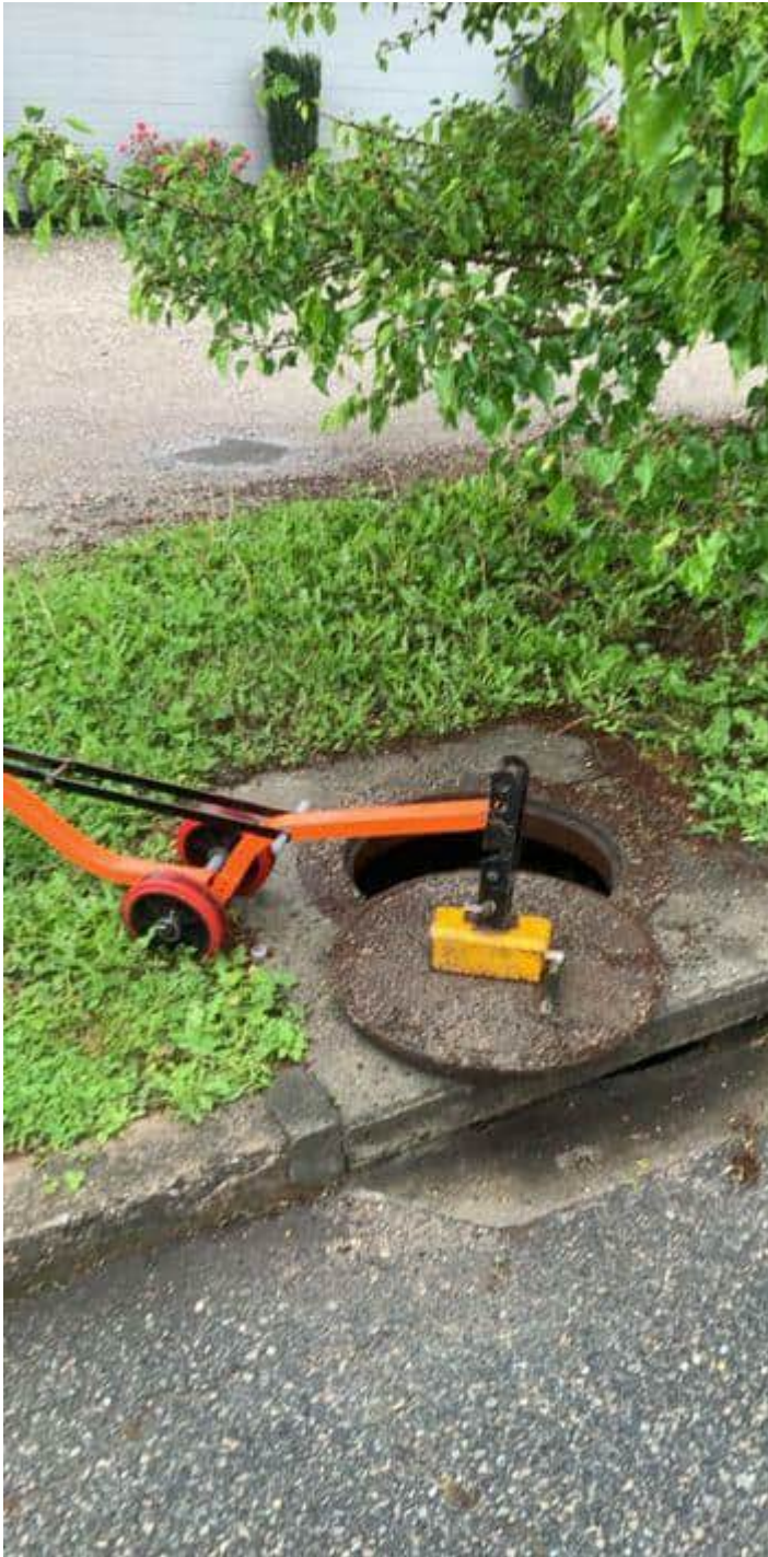
Outside pretreatment sump
