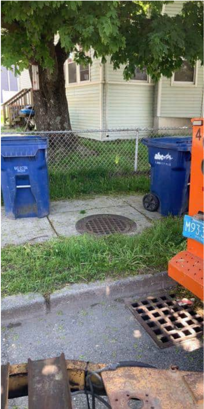
Outside tree box filter
