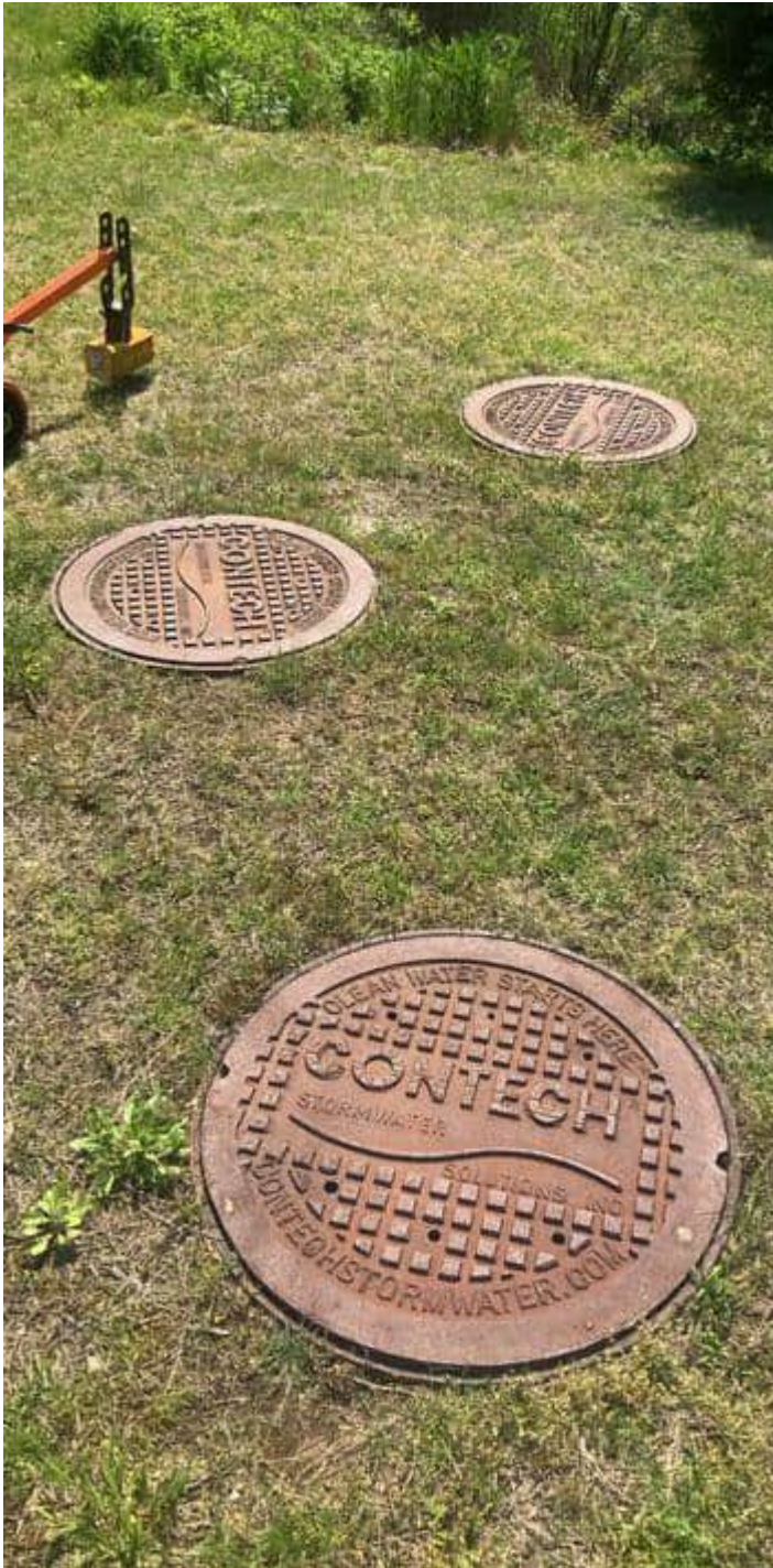
Outside water quality unit
