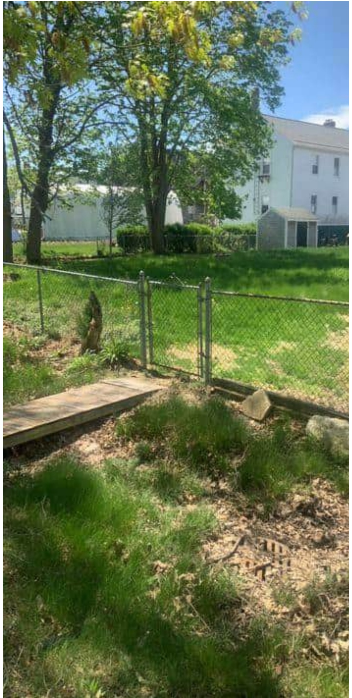
Leaching catch basin in swale
