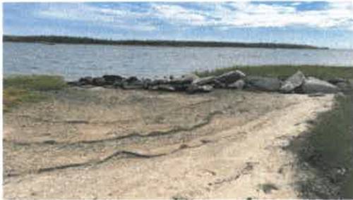
Photo 2 – East-end riprap close-up at low tide (undermined toe visible).
