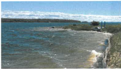
Photo 3 – East-end riprap at high tide under north wind (nearly overtopped).
